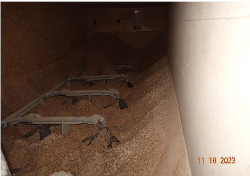
Pelletspeicher in Garage
